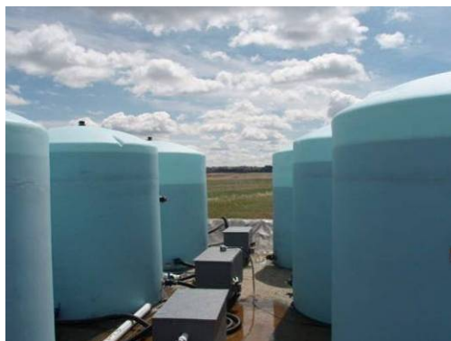
FIGURE 1 The six 3000-gallon tanks full of liquid deicers at TRANSEND. Along the center line are the three pumps used to mix one tank of each deicer.
