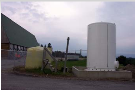
Old 2,000 gal tank (yellow) and new 10,000 gal tank (white)
